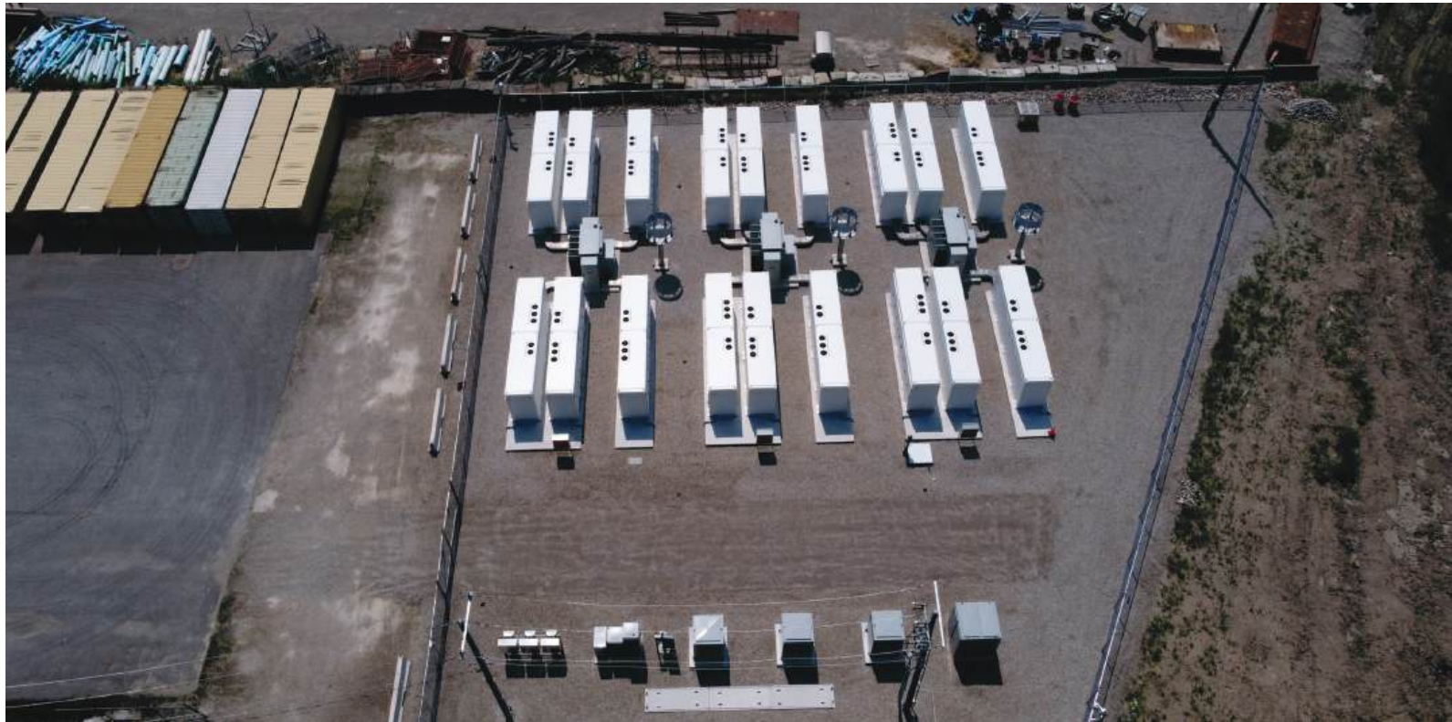
Example of a BESS Project under operation – Compass Greenfield Development’s Walker BESS 4, 5 and 6 (3 projects, 15MWac total), located in Windsor, Ontario.
